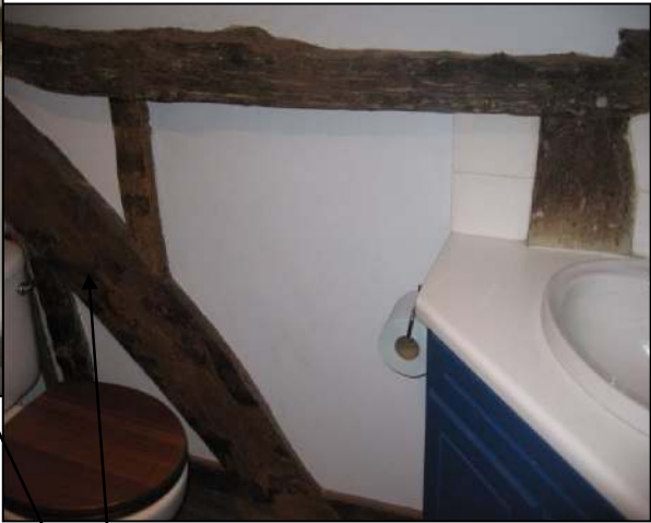
Long arch brace seen in two parts on the stair landing and in the rear bathroom.
