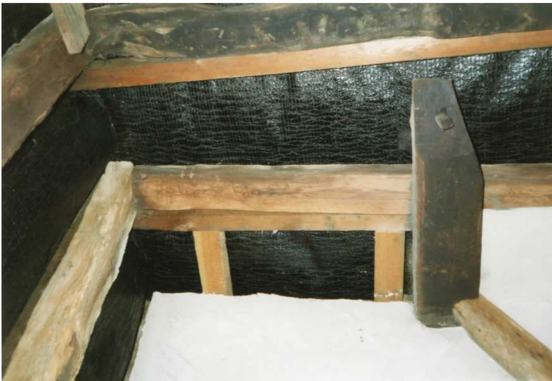
Below: Part of a Purlin is projecting from the Loft of No. 17 This and some of the Rafters are Smoke-Blackened
