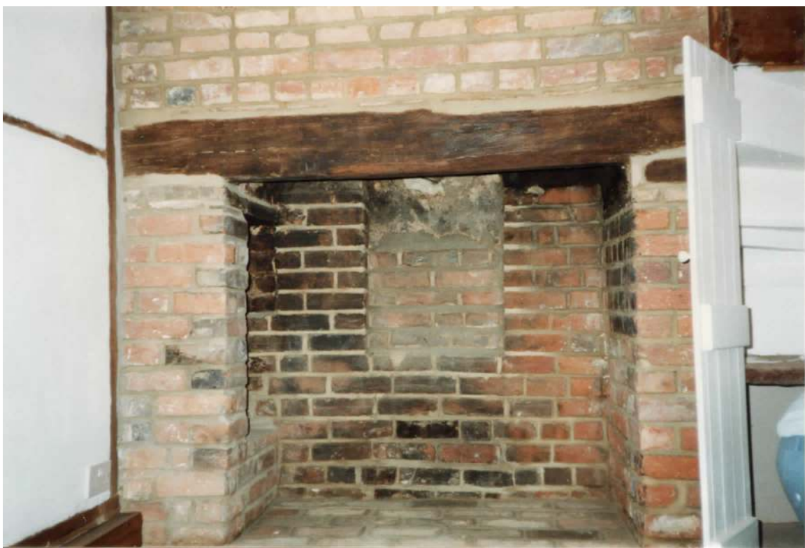
Fire-Place in Ground-Floor Front Room of No. 19 - Cleaned and Restored during present Renovation Work -
