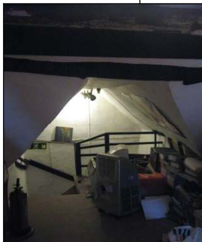
View of turned stairs at the back of Bay II. Access was gained into the attic by the removal of most of the rafters at the back/west side of Bay II of the roof. One of the horizontal timbers was probably the purlin, but additional timbers seem to have been added to make up for the loss of a large part of the rear roof of the central bay.
