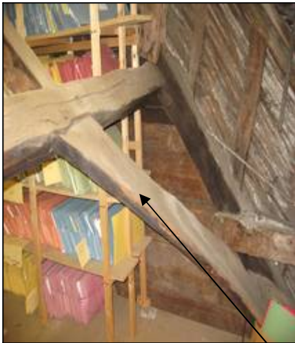
Medieval roof with purlin and wind brace preserved under the modern, shallow pitched roof of the front/east elevation. The medieval timbers are sooted, a sign of the use as an open hall of at least two bays of the building
