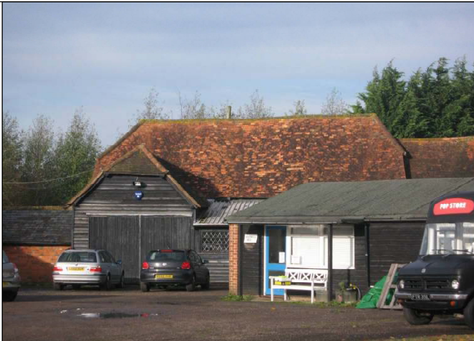
South front of three-bay timber framed and weather boarded barn with porch and half hipped, tiled roof. The lean-to, just visible behind the modern shed, appears to be a later addition or a re-built animal shelter shed, often found attached to the exterior of barn walls on Chiltern farmsteads.
