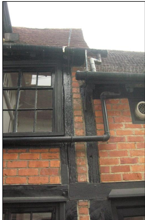
External view of the two structures, separated by a gap of c. 12 cm, now infilled with header bricks.
