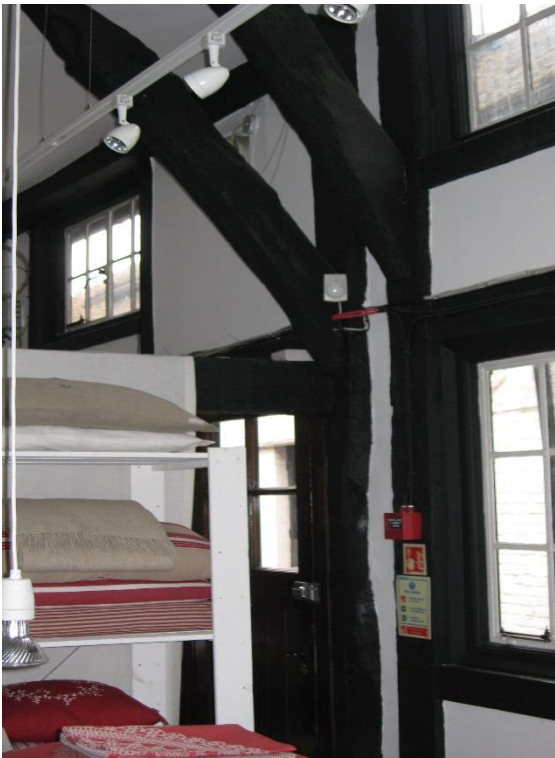
West wall with two separate trusses of bays II and III. Both have long arch braces between wall posts and tie beams
