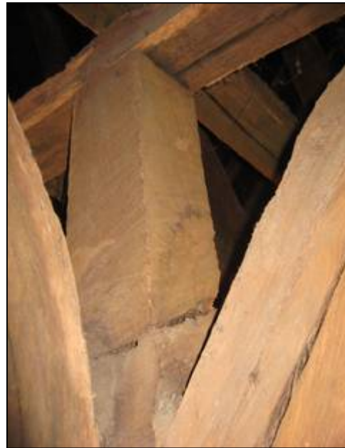
Square shaft with deep crack above capital. It still supports the 4 braces & collar purlin.
