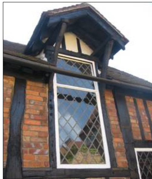
The former hoist door, now a high window. This appears to be a later insertion. The window is C 20 th as are all other windows.
