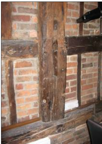
The south wall post of Truss C showing a brace slot and empty mortise of a former rail dividing the room.
