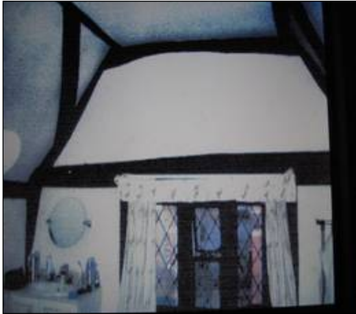
1 st Floor chamber, Bay I a on plan. Tie beam and collar only visible
