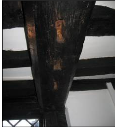
G.F. transverse joist between Bays V a and V b, formerly divided into two rooms.
