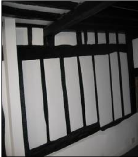
G.F. south range, south wall, Bay V a on plan. The ceiling beams support an impressive 1 st floor chamber
