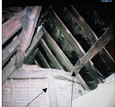
Attic above Bays II a & b, with the crown strut rising from the here hidden tie beam to the cambered collar. The purlins are clasped between principal rafter & collar.
