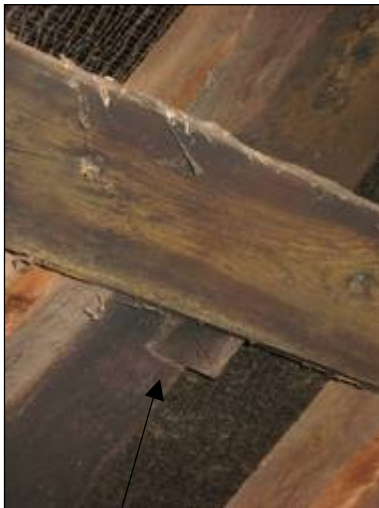
Rafter extension in 1590 through a simple lap joint for the new, taller roof. NB still smoke blackend
