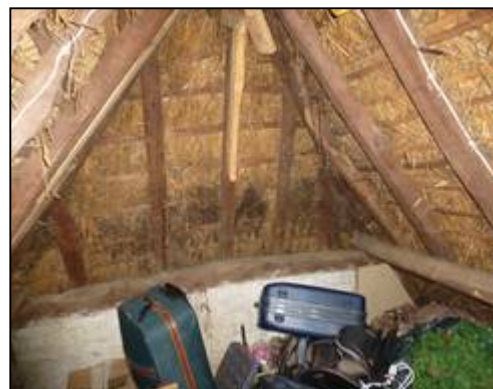
Attic of Bay III view of hip, which may be a rebuild or heavily repaired.
