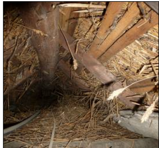
View into roof space above Bay II showing ridge beam, narrow rafters, long-straw base coat of thatching
