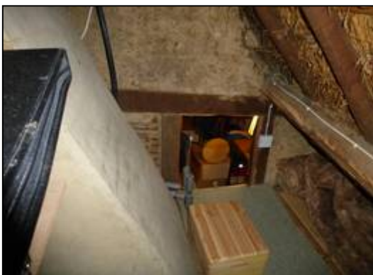
Attic of Bay III, rendered brick stack in the foreground. NB floor is higher than that of Bay II.
