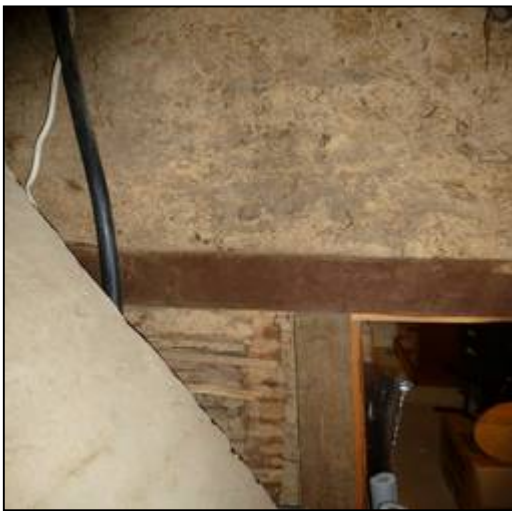
View of north facing queen strut truss in attic of Bay III; NB no weathering of collar or struts
