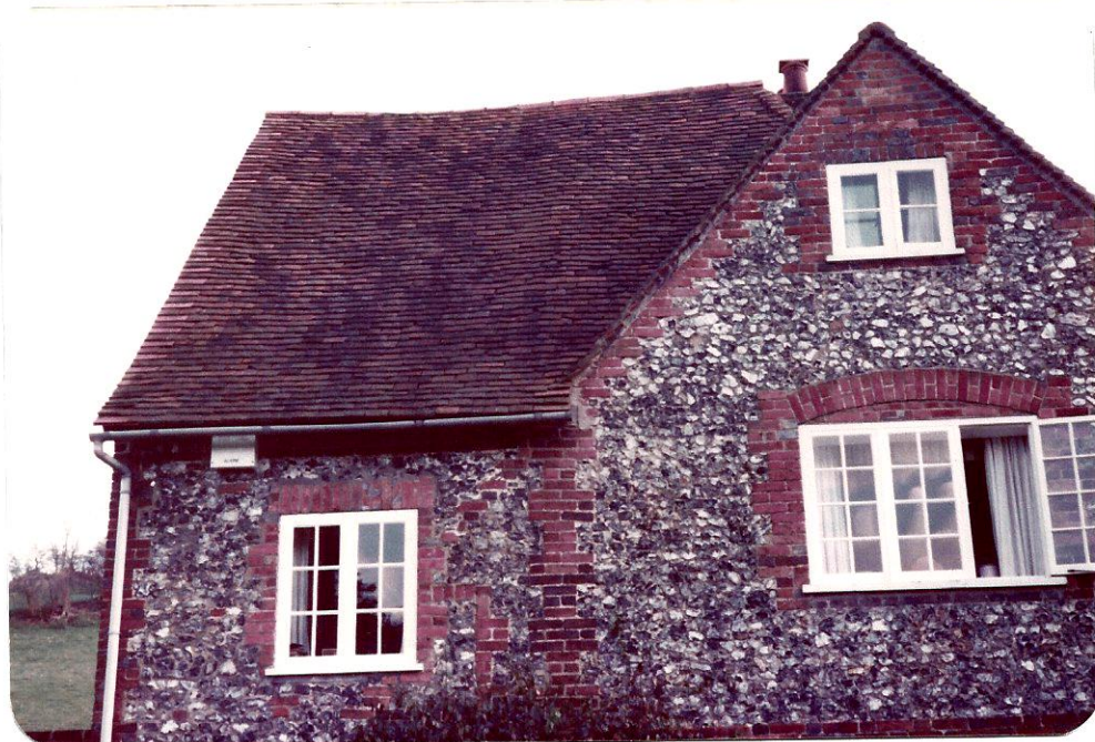
West side. Brickwork in 18th cent. part ( on the left-hand side) shows the existence of an outshot before new part was built up.
