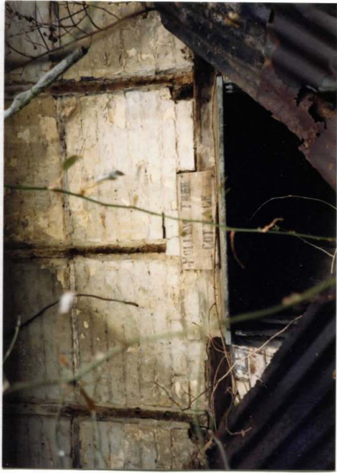
Entrance with collapsed porch
