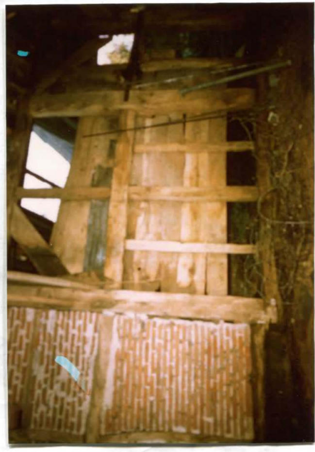
Wall between trusses F and E (brick) and E & D (timber). Note low wood-sill
