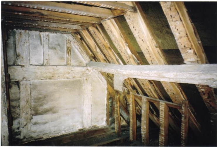
View of north end gable wall in attic of what is now No.95. NB no other equivalent of the original framing of a cross or end wall survives in the building.
