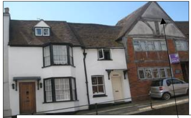
No. 9 No. 11 No. 13 NB different roof heights of Nos 9 and 11 Original 1454 crown strut roof truss
