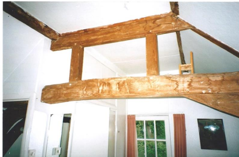
View of the queens truss on the first floor of the rear wing
