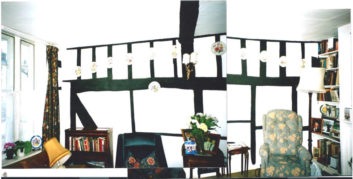
Front room, north wall shows the framing of a medieval house; a jetty is indicated on the left hand side. None of the original framing of the front wall survives, as this was removed when the building was re-fronted in brick.
