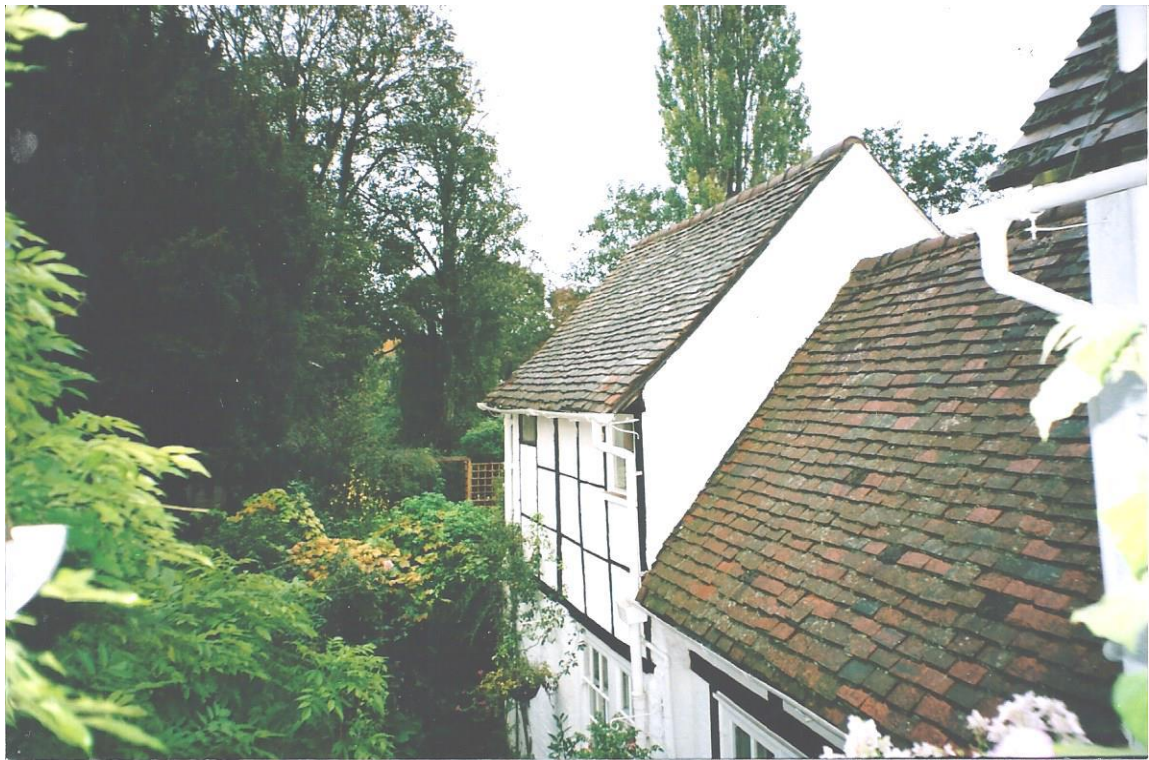
View of the rear wings. The nearest roof is that of the medieval hall. The taller, two-storey building is of slight scantling and probably of early 18 th century date. Traditions has it that it was used as a stable.
